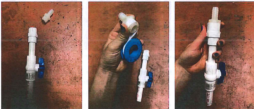
Figure 11. Gas Pipe. November 23, 2019.
